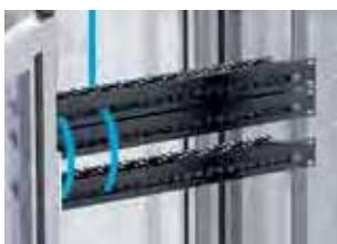
Components for the Floor Distributor
